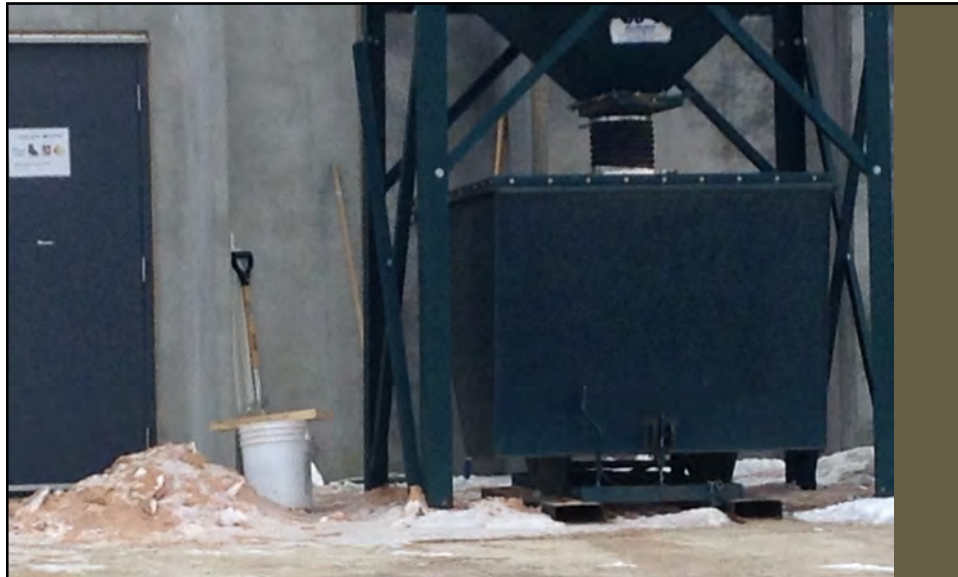
G - Containers of materials or products which are deteriorated or leaking; containers without proper covers or secondary containment I - Waste material in uncovered disposal areas, open dumpsters or open roll off containers
