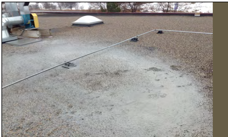
K - Visible deposits of particulate matter or residuals from roof stacks and/or vents or other sources and evident in the stormwater runoff
